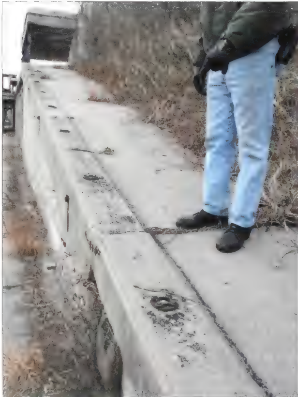
Figure 5.49. View looking northwest at the concrete ramp to gun platform #1, Nine Gun Battery. New safety railings should be installed on the ramp to facilitate visitor access. The rails should either attach to the existing escutcheon plates or be core drilled into the ramp's concrete structure. The new handrail components should match the original pipe railings and ball joint connectors at Nine Gun Battery to the greatest extent practicable (Olmsted Center, January 2009).
